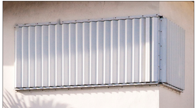
Solid metal louvers obscure windows and are not appropriate at historic buildings.
