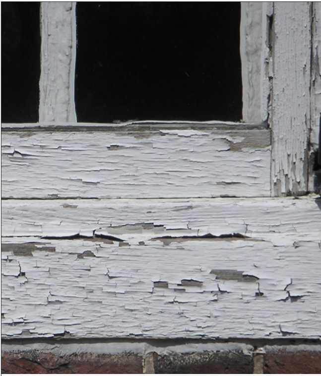
The window sill and jamb have peeling paint and some checking or splitting. Removal of the loose paint will allow the wood to be inspected for signs of rot.
