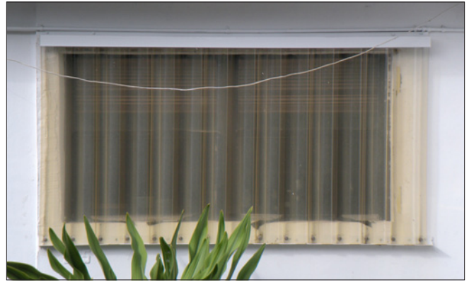
The corrugated Plexiglas in this example has yellowed and obscures the window. It is not appropriate at a historic building.
