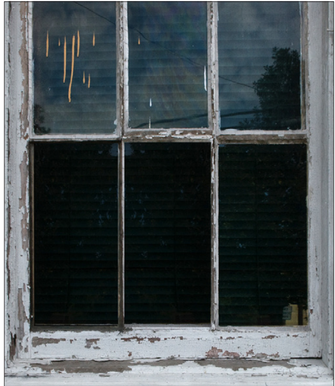
Often, the deterioration of wood windows first occurs at the sill. Peeling paint can allow moisture to enter wood and cause rot. Regular repainting is recommended to provide a protective layer against moisture.
