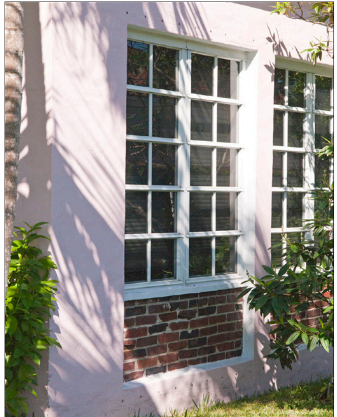
The small holes along the top and bottom of the window allow quick installation of fabric storm panels and are visually inobtrusive.
