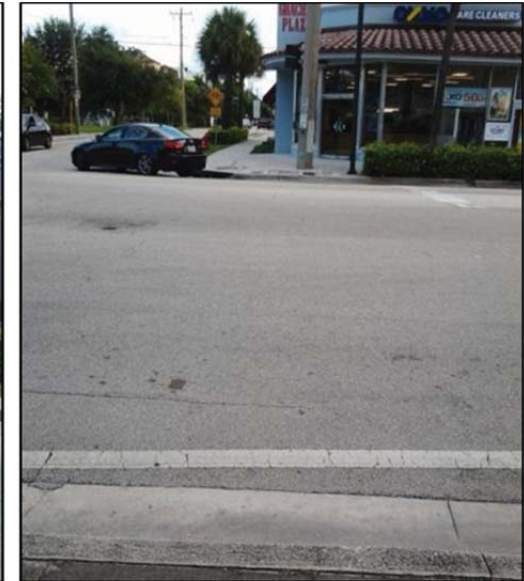
Missing Crosswalk across Las Olas
