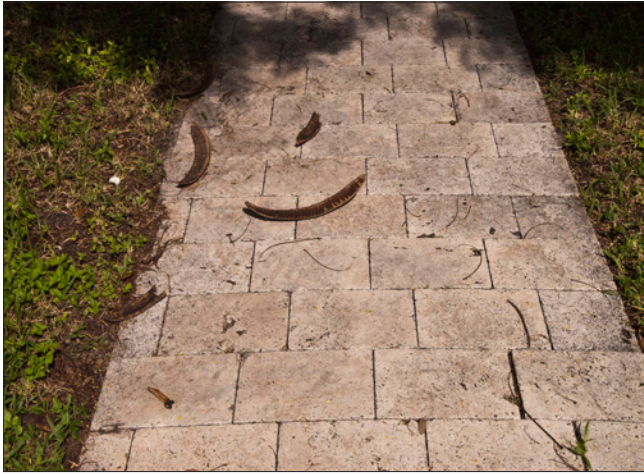
A variety of materials can be used for walkways including stone. The stone paving in this example is a local limestone known as oolite or keystone.
