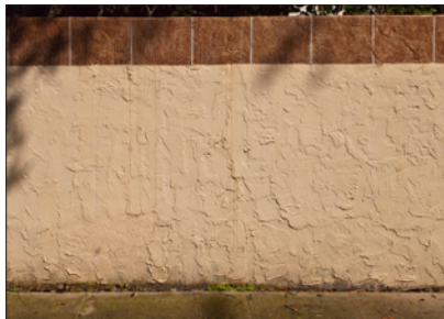
Most landscape walls in Fort Lauderdale are stuccoed, with the color and texture generally complementing the principal historic building.
