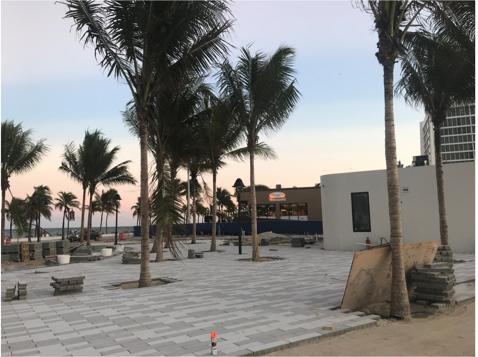
OCEANSIDE PARK PROGRESS PHOTO TAKEN ON 10-15-19 (PAVER INSTALLATION – EAST SIDE OF PARK)
