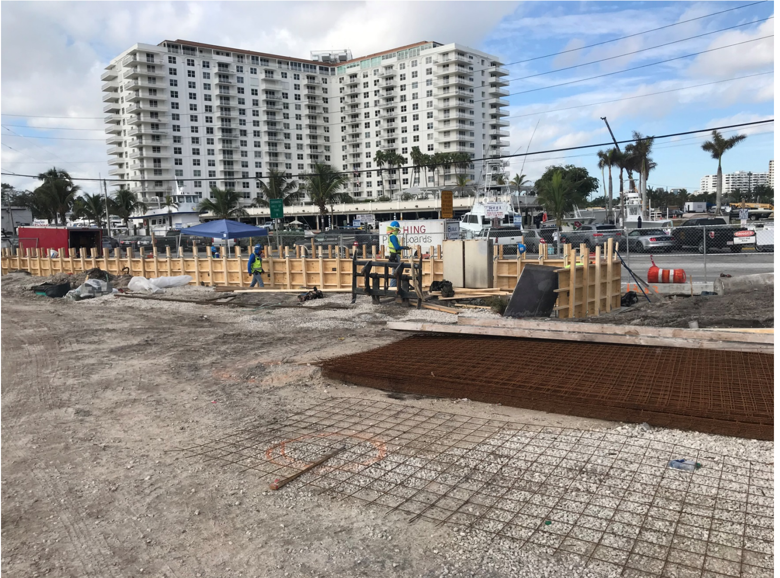
OCEANSIDE PARK PROGRESS PHOTO TAKEN ON 10-15-19 (FORMING RETAINING WALL – WEST SIDE OF PARK)
