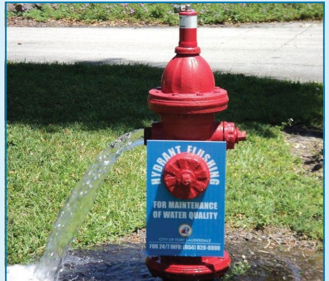
Flushing fire hydrants is a routine part of the free chlorination process.
