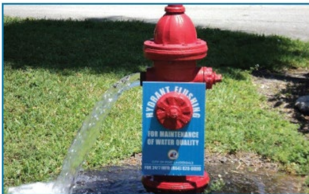
Flushing fire hydrants is a routine part of the free chlorination process.
