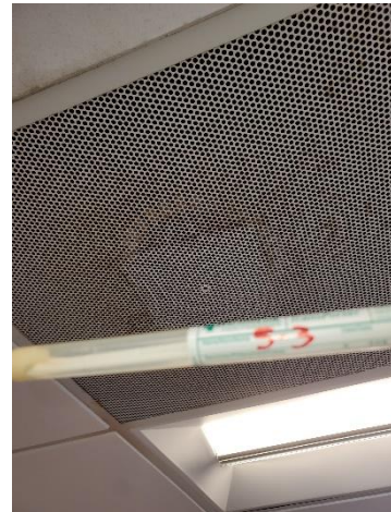
Photo 4: View of a representative supply air diffuser.
