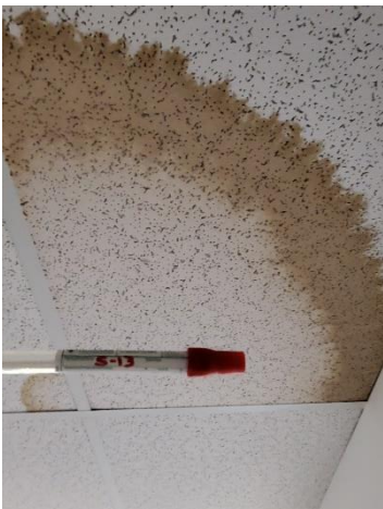
Photo 5: View of water stained ceiling tile – 2 nd floor south cubicle area.
