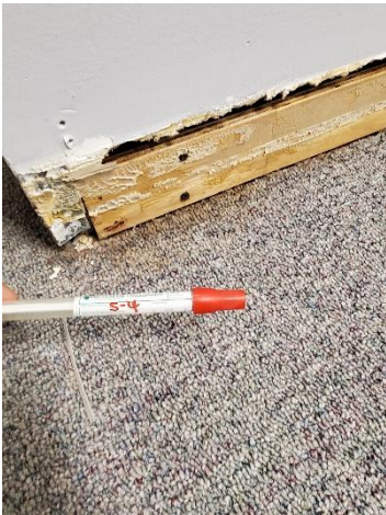
Photo 3: View of stained carpet – 7 th floor.
