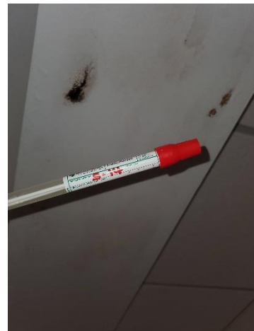
Photo 6: View of 1 st floor - stain hard ceiling.
