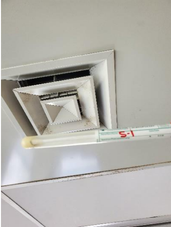
Photo 1: 8 th floor conference room A/C supply.
