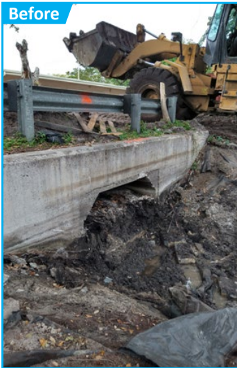
Melrose Park Drainage Culvert: Clogged with Tropical Storm Eta sediments
