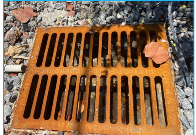
Fort Lauderdale Catch Basin
