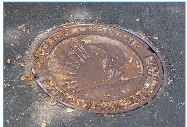
Fort Lauderdale Manhole Cover
