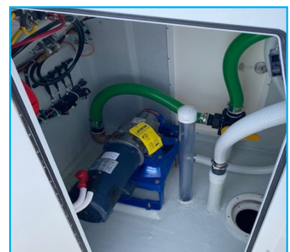
Marine Boat Builders Co. integral on board pumpout system
