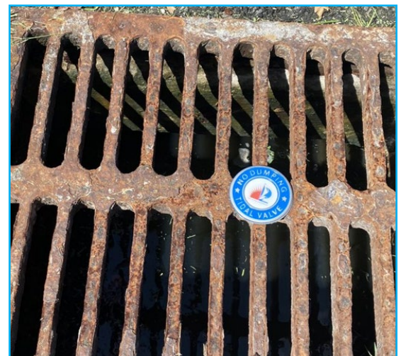
Figure 2 - Storm Drain with a tidal valve installed. Only the last storm drain before the discharge point is a candidate for a tidal valve and most of the 185 catch basins with a tidal valve are marked with a medallion.
