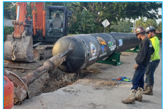
Preparing to pull the pipe back through the Horizontal Directional Drilling hole
