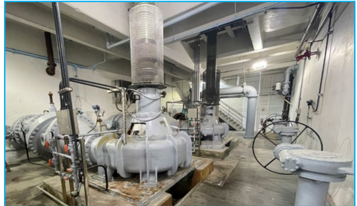
Injection well pumps at George T. Lohmeyer Wastewater Treatment Plant
