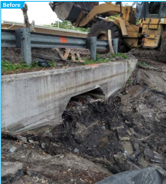
Melrose Park Drainage Culvert: Clogged with Tropical Storm Eta sediments
