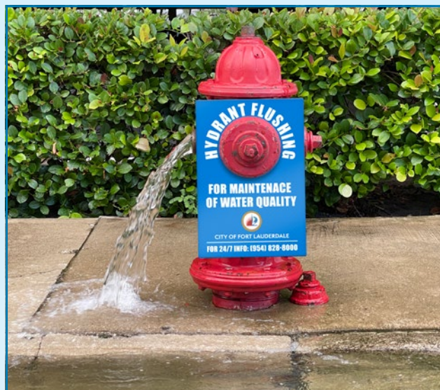
Flushing fire hydrants is a routine part of the free chlorination process.
