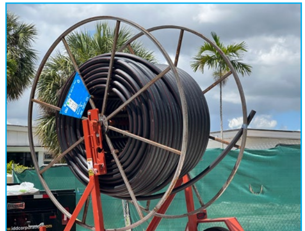
Conduit used for underground FPL lines
