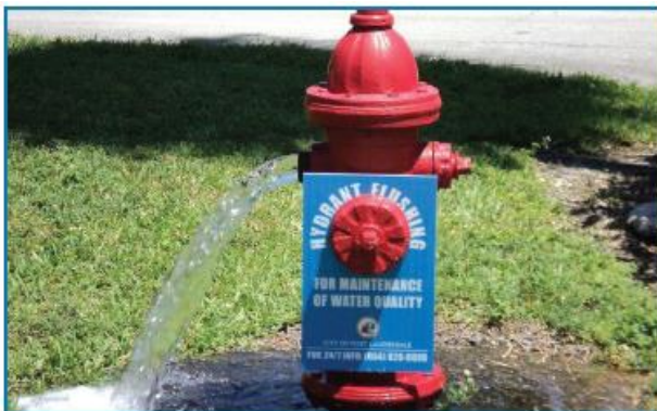
Flushing fire hydrants is a routine part of the free chlorination process.
