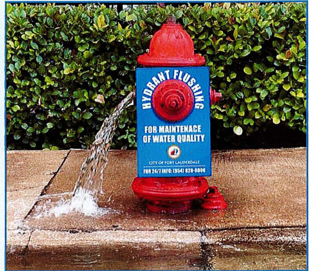
Flushing fire hydrants is a routine part of the free chlorination process.
