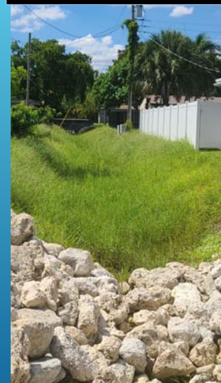
Drainage ditch becomes re-established
